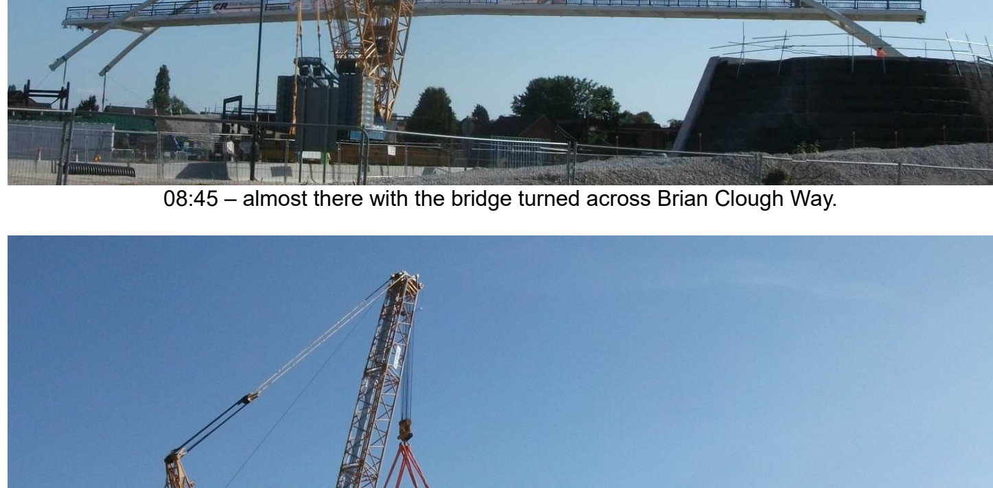
08:50 – being lowered onto its permanent foundations. Hope it is the right length!
