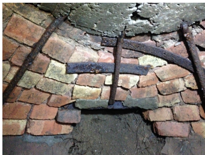
Fig. 4: This photograph was taken a little to the right of Fig. 3 and clearly shows the concrete roof cap as well as a recess in the wall of the chamber.
