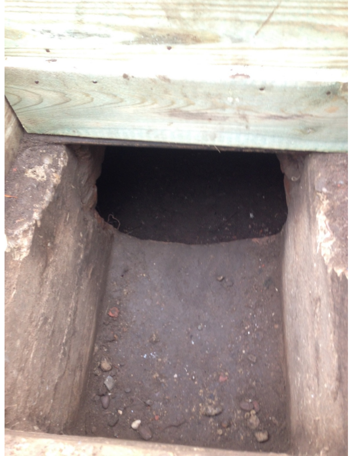
Fig. 2: This brick-lined cavity was revealed when the hole was cleared out. Note the start of the much larger void at the back.
