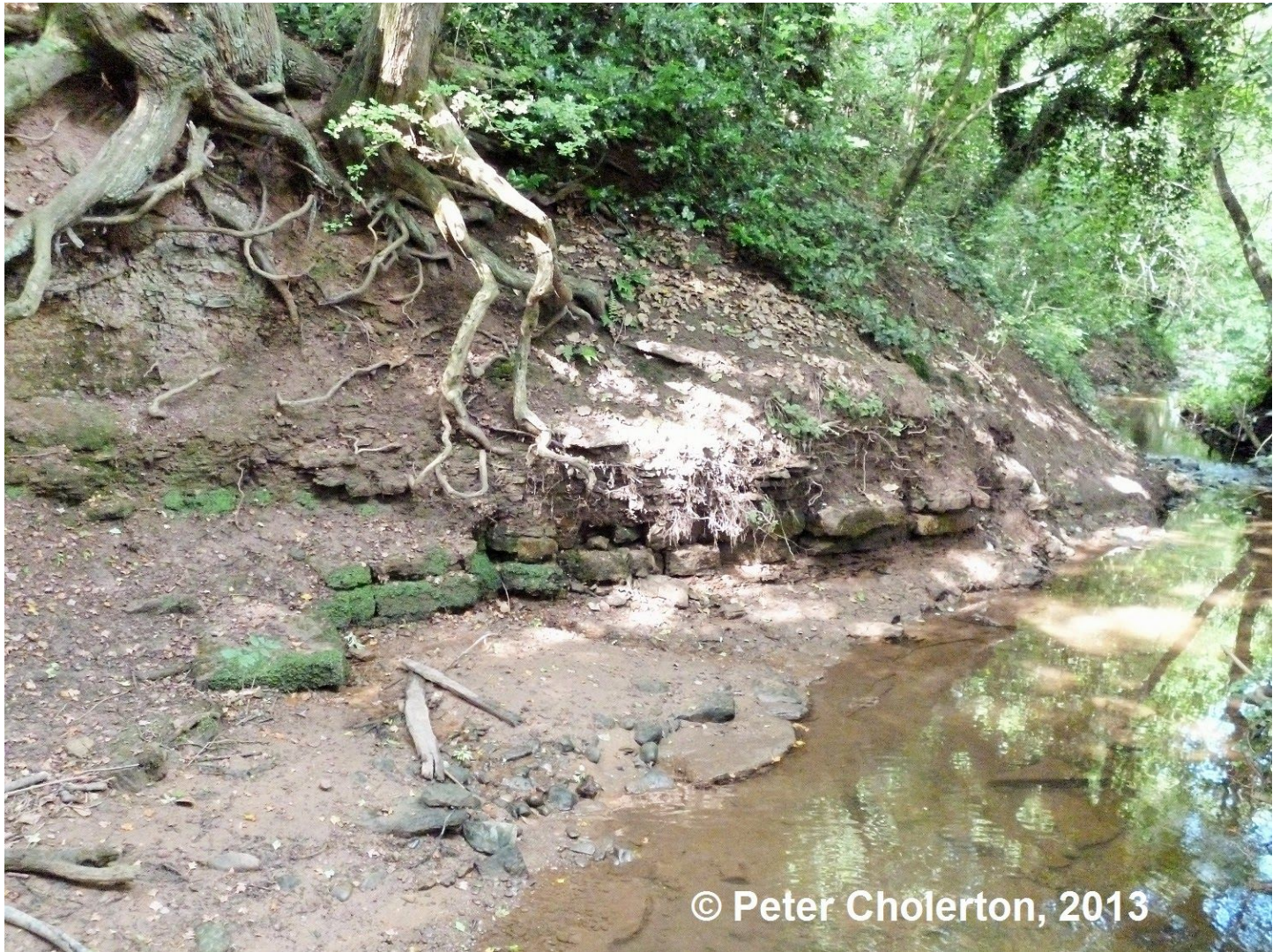
Fig. 6: Partly obscured by tree roots and vegetation, this section of dressed stone walling on the south side of Lees Brook some 20 feet below the surrounding ground level might once have been associated with Bradcar Watermill. Photographed on 9 August 2013.
